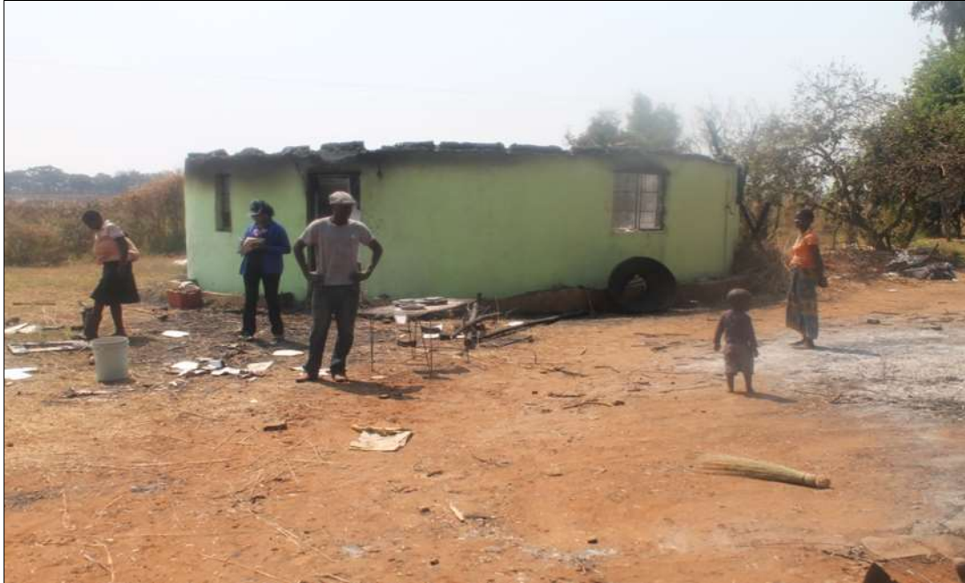
Plate 8: Farm house gutted down by veldt fire at Hargley Estates in Lalapanzi area of Chirumanzu district.
